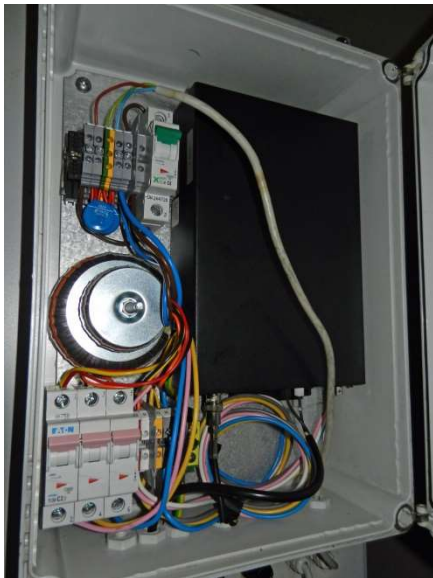
Vestas Telecom with fiber optic
